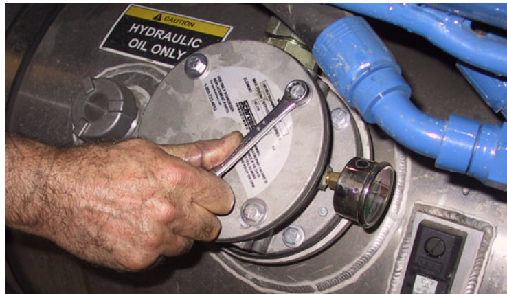
Figure 7-15 Loosening plate bolts
